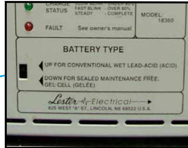
Close up of dip switch
