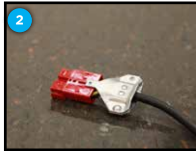
Anderson connector located on charger cable
